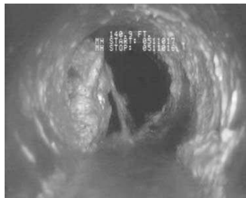
Partial grease blockage in sewer pipe
