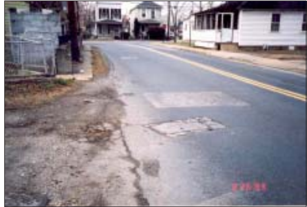
Much of the community's infrastructure is in need of repair.
