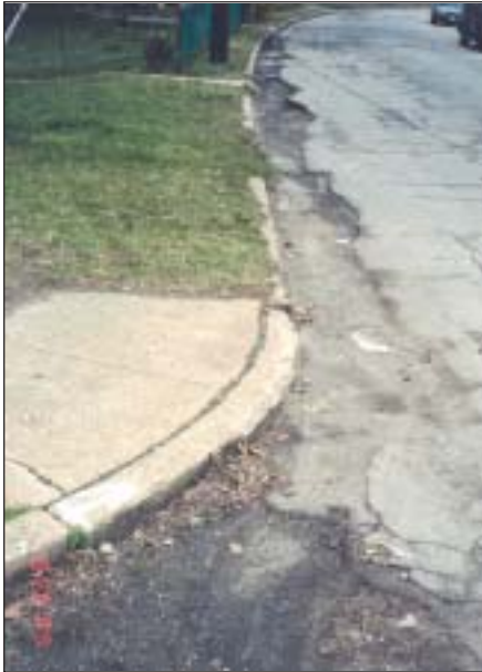
Sidewalks in many locations are deteriorated or non-existent.
