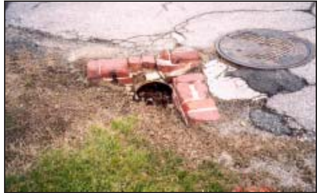
Storm drains in neighboring Carnegie Platt are in need of repair.
