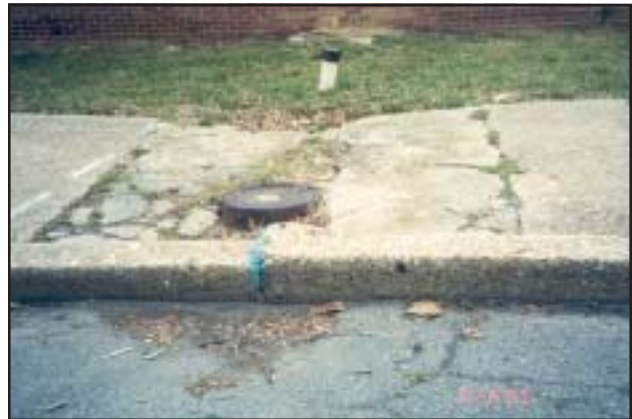
A deteriorated storm drain located on South Lane.
