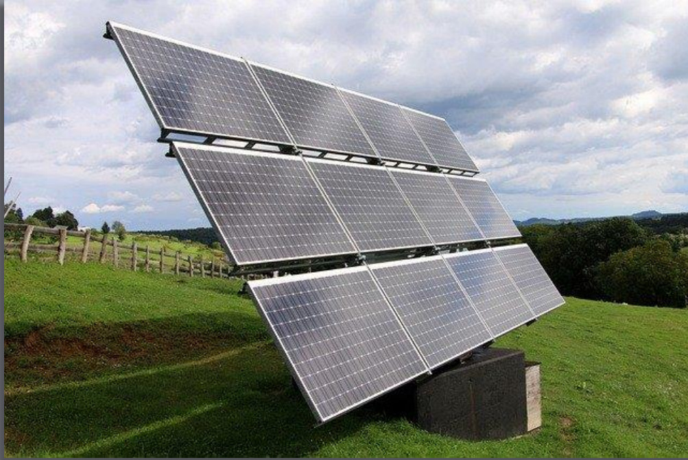
HERNWOOD AND PARKTON LANDFILLS Brown field solar
