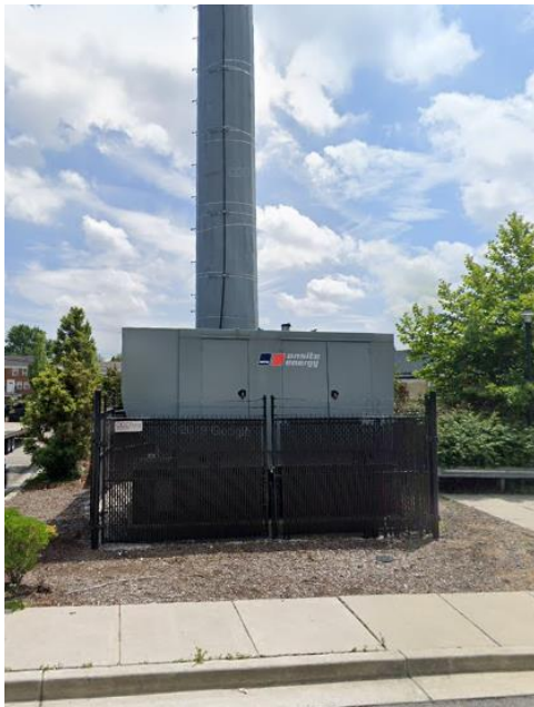
Figure 4-2: Backup Power is a Common Adaptation for Critical Infrastructure (shown at a cell tower)
